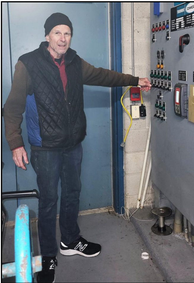
Head ice technician Jeff Gray turns off the plant for the last time.
